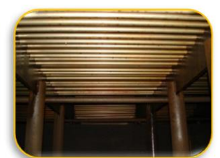
Chemically Cleaned Condenser Tubes
