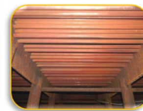
Rusted Condenser Tubes
