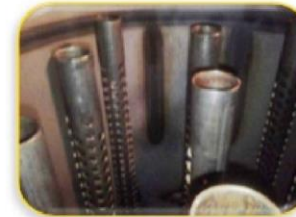
Filter Housing After Varnish Mitigation Service
